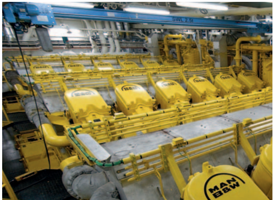
Engine Room Crane SWL 2.5t Class LR
