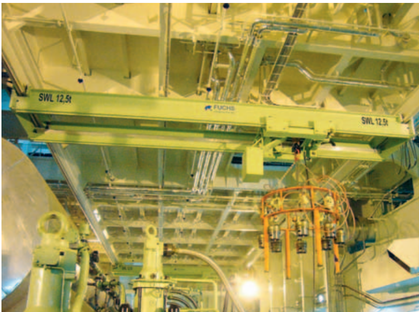
Engine Room Crane SWL 12.5t Class LR
